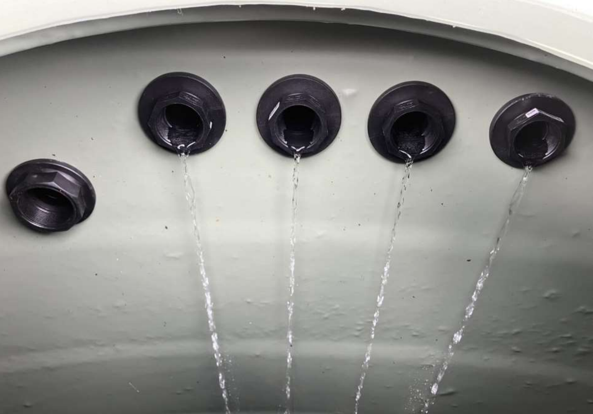
November 2023 - Water flow from each well coming into the header tank
